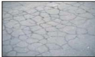
Fatigue (Alligator) Cracks
