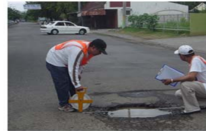
2. Measure longest diameter of the pothole
