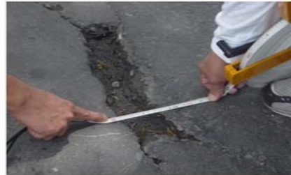
4. Measure largest width of crack
