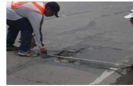
4. Measure length of largest crack
