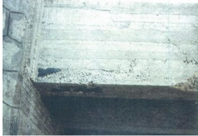
Honeycombing is an indicator of poor quality concrete
