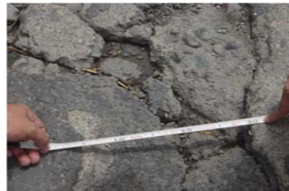
4. Measure largest width of crack
